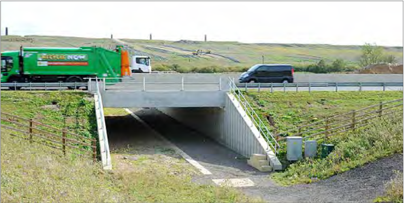
Both sides of the underpass – the part that will become the waterway and the part that will become the foot-and-cycleway – have been filled with loose earth (for safety reasons) and lights provided along the tunnel.
